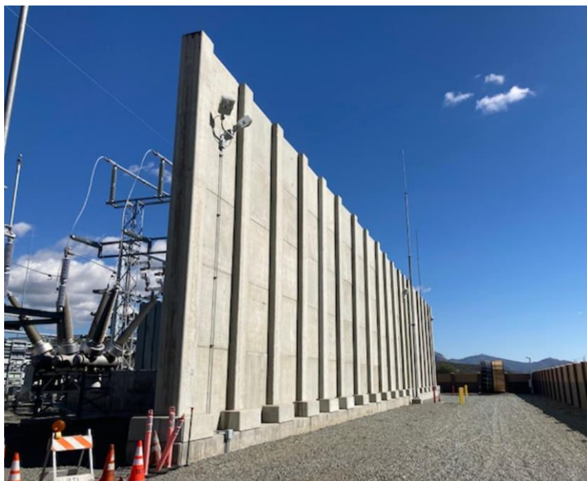
Figure HWT 8.1.2-1. Transformer Fire Barrier Wall
