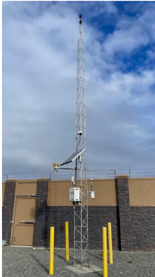
Figure HWT 8.3.2-2. Weather Station
